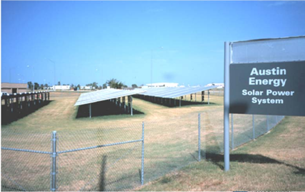
Large generation systems connected to the Grid
